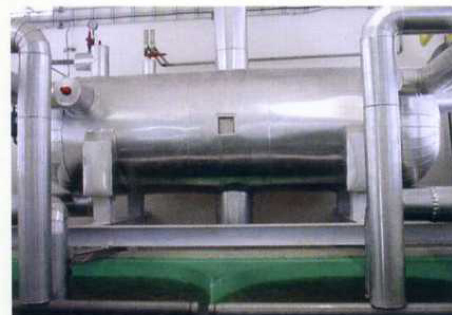
Liquid Separator Vessel
