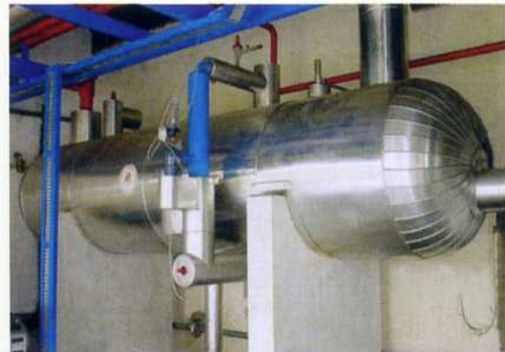
Horizontal Intermediate Cooler Vessel
